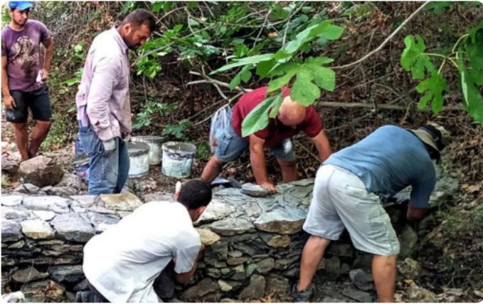
Construction of a micro-dam with local stones, near Karavas village on the island of Kythira, Greece
